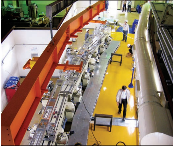
A 14-m long "hanger", equivalent in size to the vacuum chamber, was built to carry the assembled unit.
