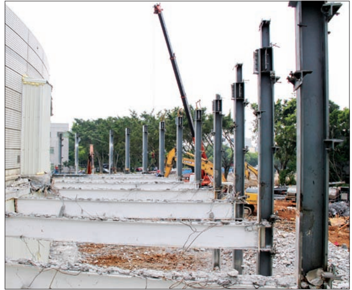
Walls of the TLS building were torn down for the new interface with the TPS storage ring and piles were inserted to stabilize the TLS foundations.
