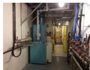
Fig. 1: Installation of the triode amplifier, visible are (a) the 3" feedline from the preamplifier on the mezzanine above, (b) the preamplifier test load, (c) the final stage amplifier assembly and (d) the 6" output line from the final stage. Image credit: TIARA/MICE.
