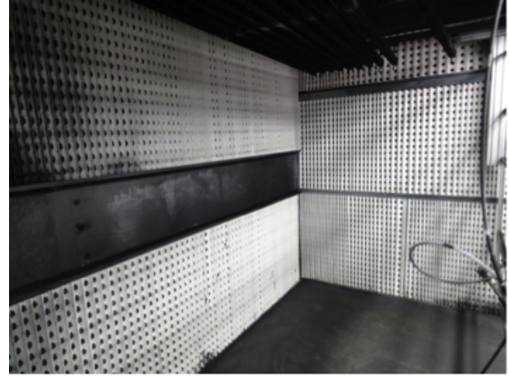
Figure 7.6: Filters and hanging rails for cathode boards
