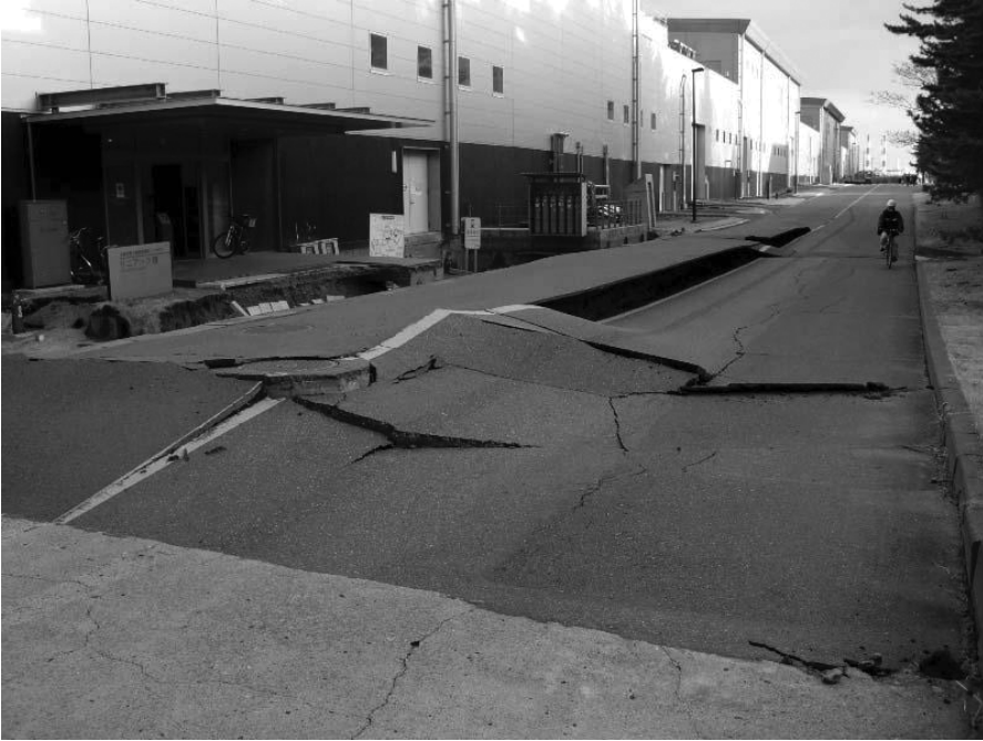
Fig. 2: Road around LINAC was completely destroyed by the earthquake. Approximately 1.5m drop of road surface was observed at wide area. Electric wires and water pipes set in the underground were all seriously damaged.
