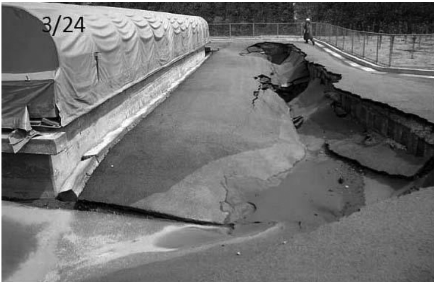
Fig. 3: At the neutrino experimental facility, ground surface around beam dump (i.e. area covered by grey tent in the photograph) seriously subsided. Beam dump itself was sustained by many underground pins and less damaged. Land around the target station subsided also.
