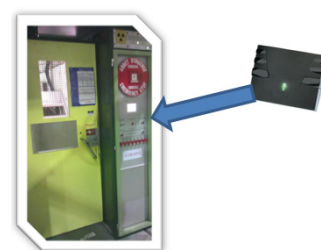
Figure 9 Addition of badge readers in AD and EH
