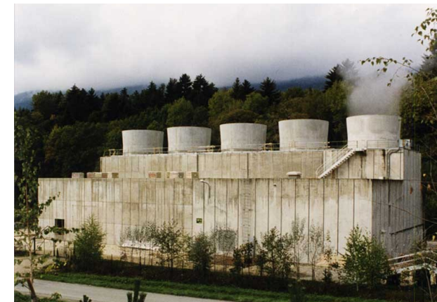
P4 Cooling towers
