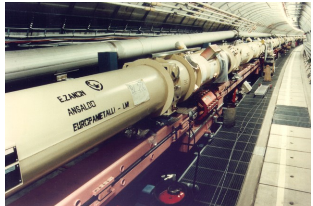
Figure 4. View of the HERA tunnel with the superconducting proton machine on top of the electron machine.
