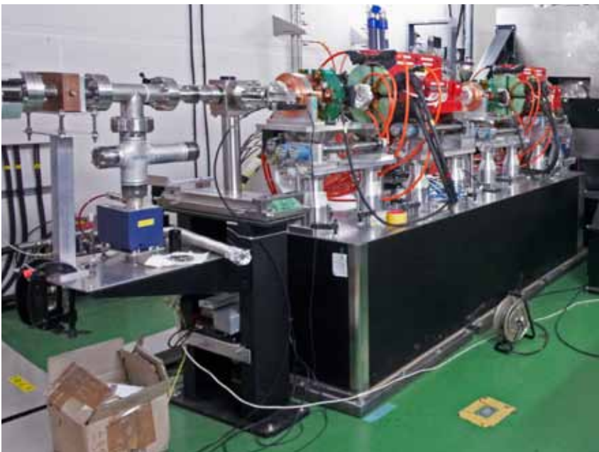
Figure 3.12 View of the final doublet installed on its rigid mechanical support system.
