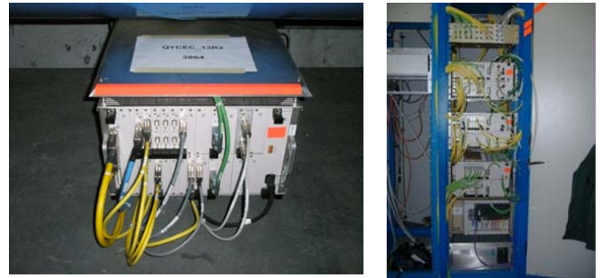
Figure 2: Instrumentation crates under the dipoles (left) and in the radiation protected areas (right).
