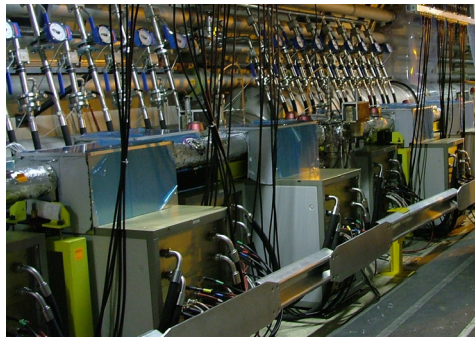
Figure 2: Kickers and amplifiers in the LHC tunnel.
