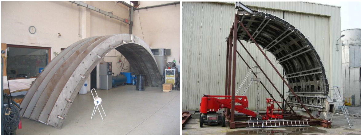
Figure 9.3: The CalFrame in the process of assembly (left) and fully assembled (right).
