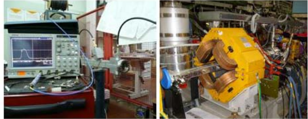
Figure 7: New fast injection kicker under test (left) and installed on the electron ring (right).
