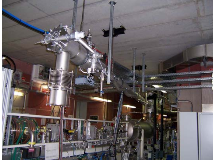
Fig. 21: Photograph of the new helium pipeline in the accelerator hall for the SRF gun
