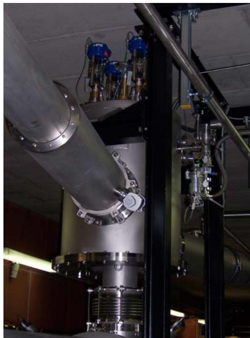
Fig. 22: Photograph of the valve box with part of helium pipeline for the SRF gun
