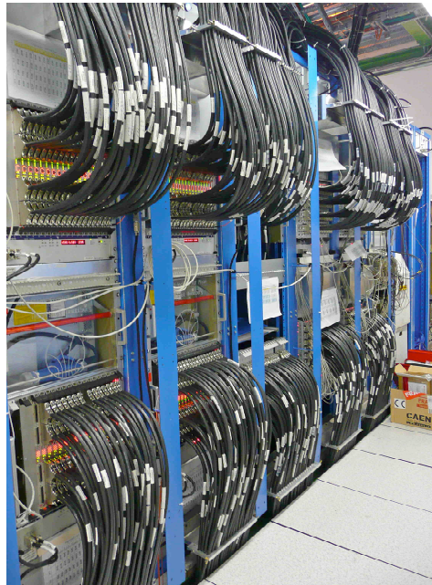
Figure 6: Short analogue cables for \eta > 0 , from Receivers (two racks at right) to PPMs (two racks at left).
