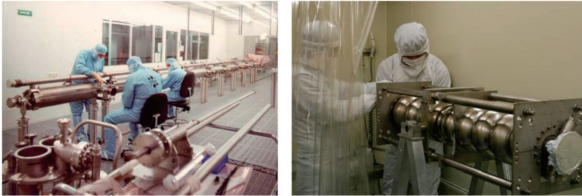
FIGURE 2.4. Clean room environments are mandatory. Left: the assembly of eight nine-cell TESLA cavities into a cryomodule string at DESY. Right: an ICHIRO nine-cell cavity is prepared for initial tests at the Superconducting RF Test Facility (STF) at KEK.
