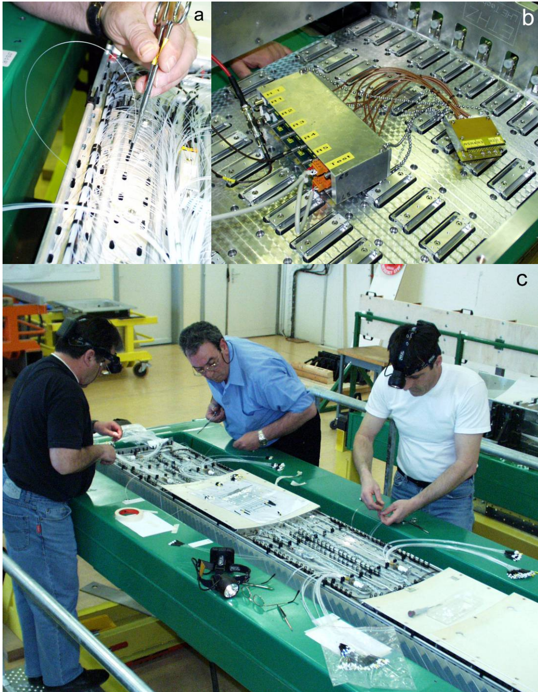
Figure 29. Installation of the monitoring distribution system on an ECAL barrel SM: (a) shows tool used to insert the optical fiber's ferrule into a crystal's ferrule support, (b) shows the 10-channel amplifier and connector used to test APD response after cabling (SM face down), and (c) shows the installation of optical fibers on alternate sub-modules (SM rotated front-face up).
