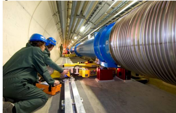
Figure 1: Transfer of a main dipole magnet on the support jacks
