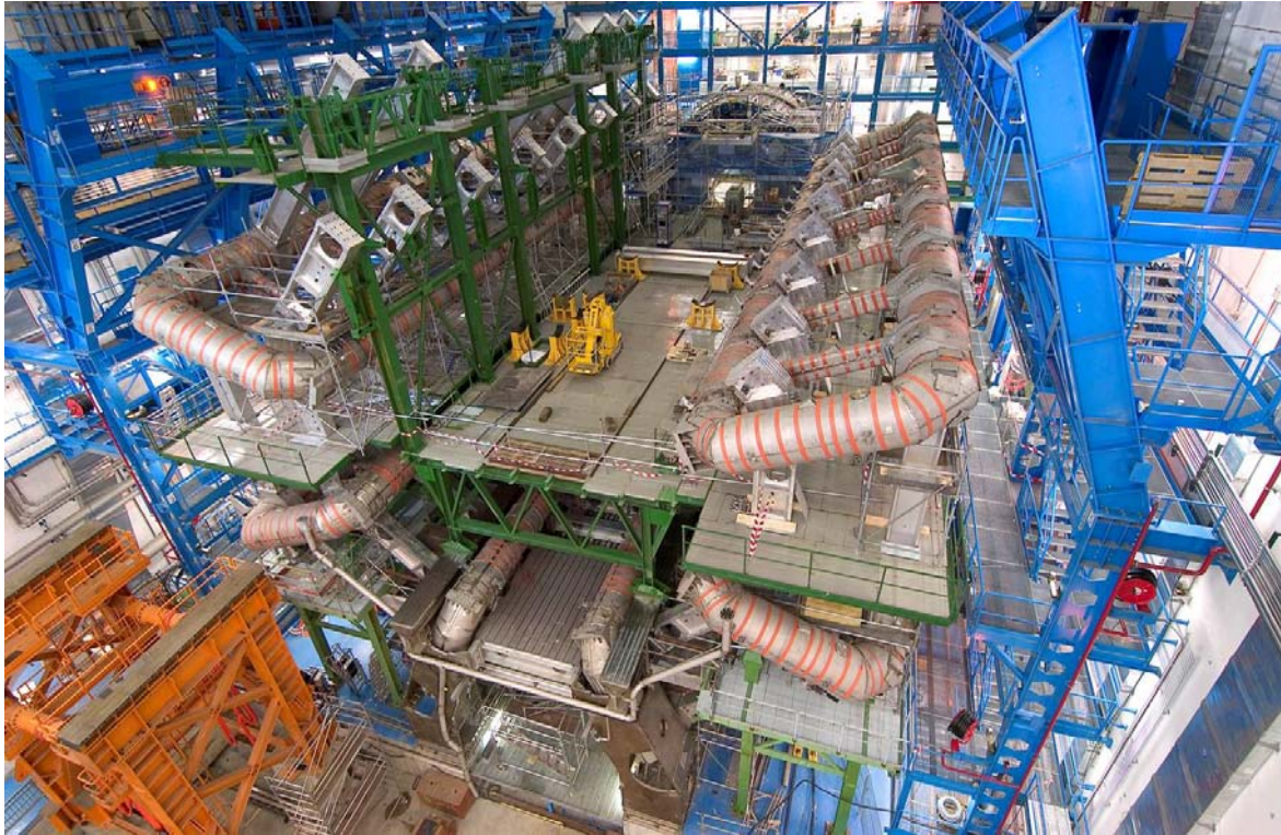
FIGURE 1. July 2005 status of the barrel toroid integration in the ATLAS cavern.
