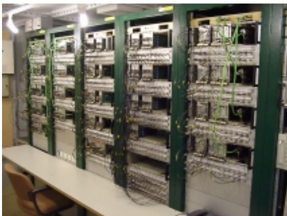
Figure 4: Electronics racks of the timing system
