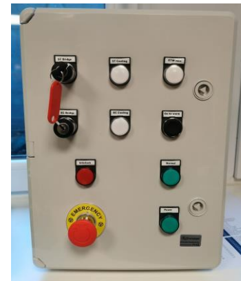
Interlock Connection Box (DESY)
