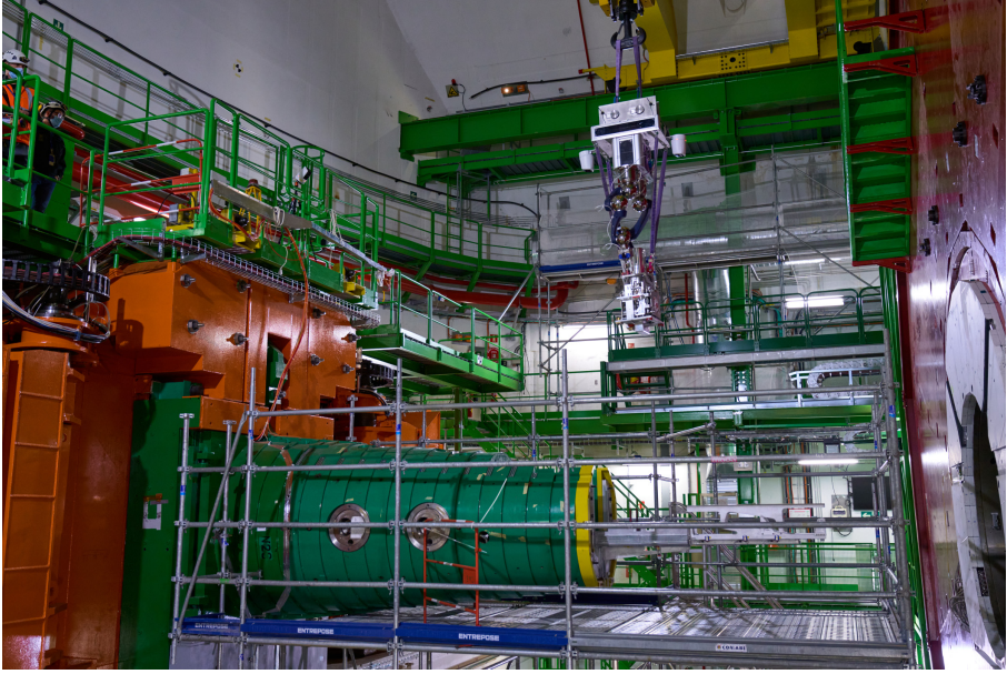
Fig. 7. The CERN CRANEbot is seen here carrying a VAX module (centre of the image) inside the CMS cavern, as part of an operation test conducted in early February 2021.
