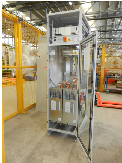
Fig. 1. In-vacuum switch based 2 kA energy extraction system.
