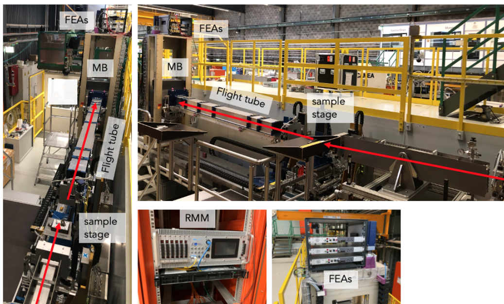
Figure 4. Pictures of the installation at Amor showing the neutron path at the reflectometer in red.
