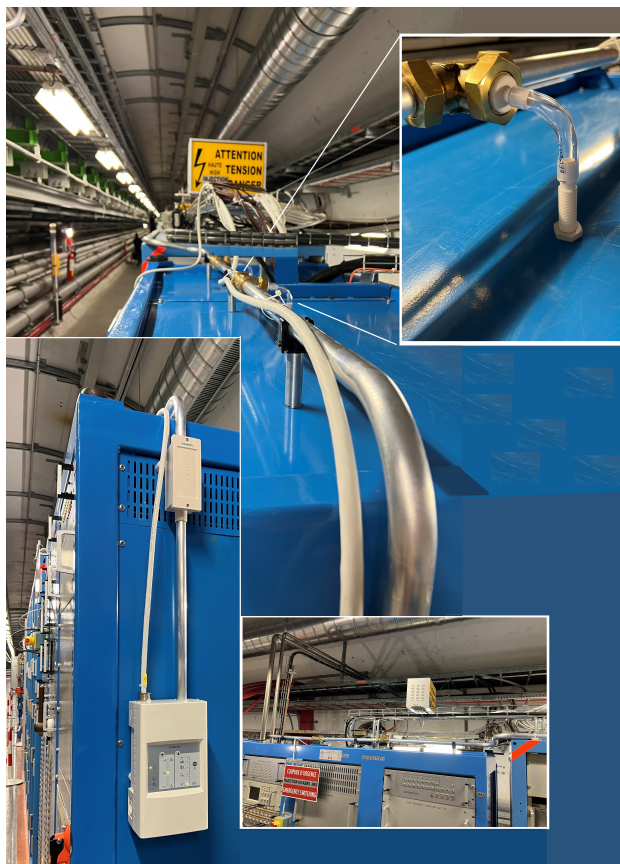
Figure 6: MKI Pipework and ASD Installation.
