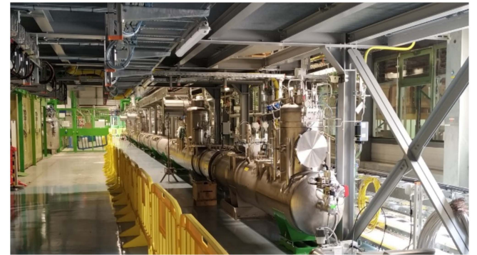
Fig. 5. SQXL, cryogenic line for the HL-LHC IT string.
