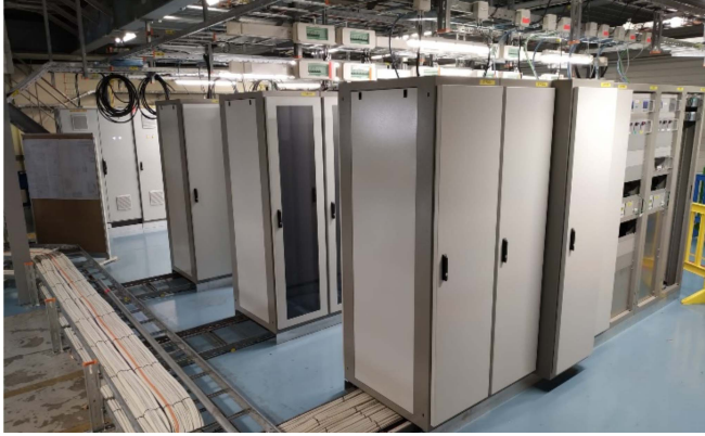
Fig. 6. Control racks of the HL-LHC IT string.
