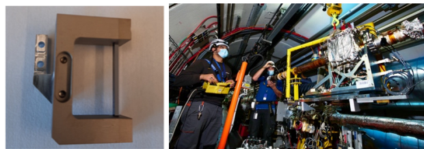
Figure 13: Left: Bent crystal. Right: Installation of new goniometer including a bent crystal in IR7.
