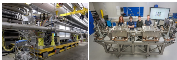
Figure 8: Left: Prototype cryomodule installed in the SPS for tests since 2018. Right: String of 2 RFD dressed cavities prior to assembly (courtesy HL-UK).
