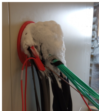
(b) Ice from air leakage
