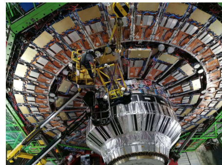
Figure 2. Installation of GE1/1 chambers during LS2.
