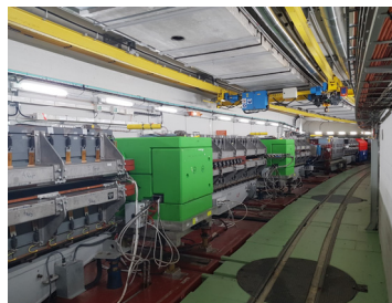
Figure 9: Photo of the PS Internal Dumps installed with their concrete shielding.
