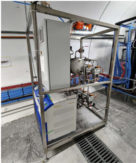
Fig. 16. Photograph of the cooling system.
