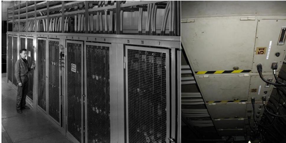
Fig. 5-15: Left: line selector in Building 251, right: terminal boxes in the technical gallery under Building 157.
