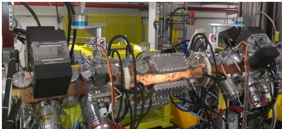
Fig. 2.4: RFQ installed in the Linac4 tunnel.
