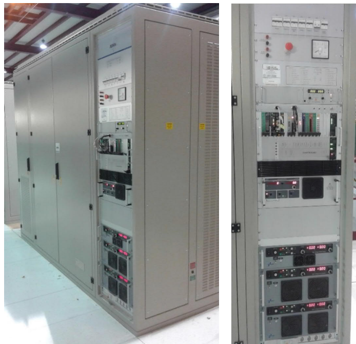
Fig. 3.32: Photo of a Modulator power converter for pulsed RF klystrons.
