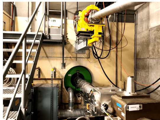
FIG. 8. View of the entrance of the beam dump cavity at the end of the BTM cavity in November 2019. Visible on the left side in the foreground under the staircase to ISOLDE, the Air Handling Unit (AHU) and the cooling ducts feeding into the cavity.
