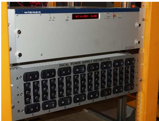
Figure 6. Photograph of a Wiener power supply with the power distribution box located underneath.
