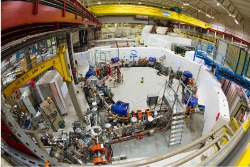
Fig. 5. The ELENNA ring and its components installed in the AD Hall.
