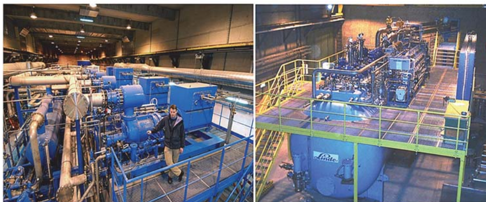
Fig. 8.12. Cryogenic plant providing 18 kW @ 4.5 K. Left: compressor station. Right: cold box.
