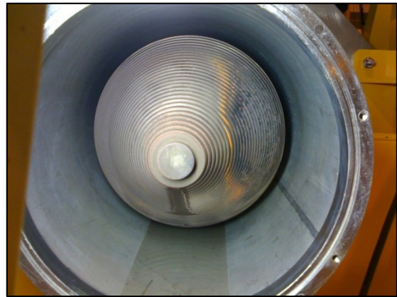
Figure 5: Klystron collector showing traces of overheating (2010).
