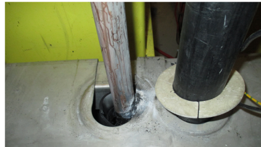
Figure 10: Photo of the QF busbar location close to QF.12010. The busbar was touching the metallic busbar cover.
