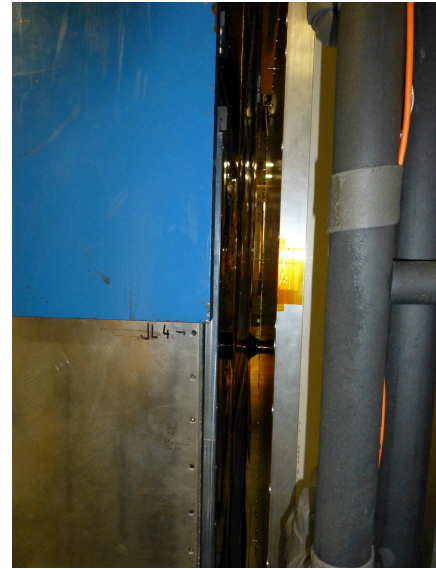
Figure 3. The VHCC between RICH1 and TT installed for Run 2.
