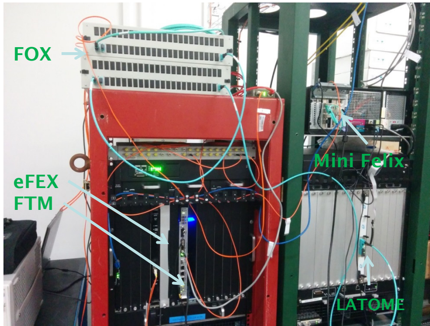
LAr LATOME AMC+ LDPB as data source @CERN (Altera Arria 10 FPGA)
