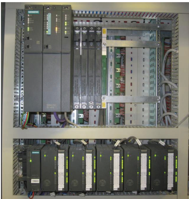
Figure 1: Siemens S7 400 series CPU with ET200 remote I/O modules.
