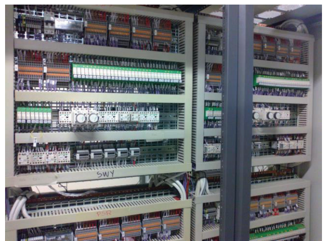
Figure 3: Hardwired relay-based logic using relays. Green LEDs indicate contact states.
