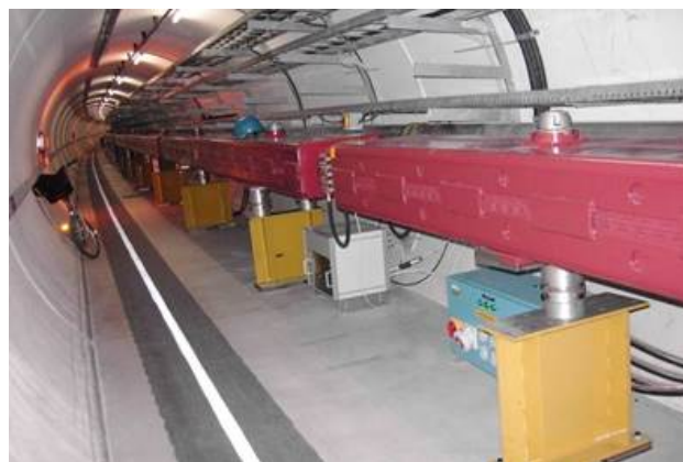
Figure 2: WIC remote I/O crate installed in the SPS Transfer Lines.
