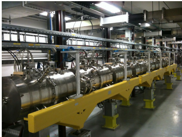
Figure 7: First 3 CCDTL modules in the Linac4 tunnel.
