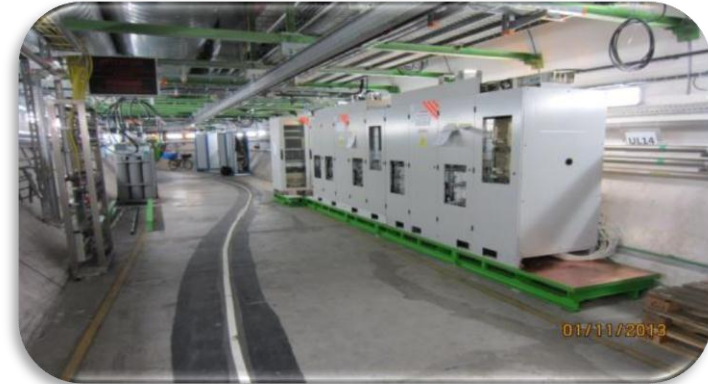
UL16 power converters
