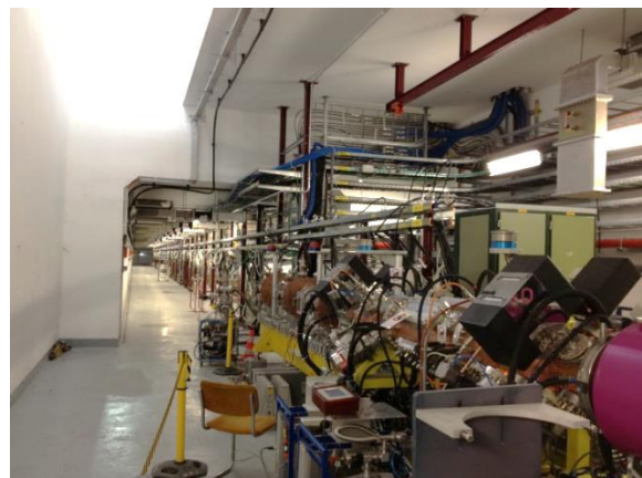
Figure 15: Linac4 tunnel seen from the low energy side. In the foreground, the RFQ and the MEBT.
