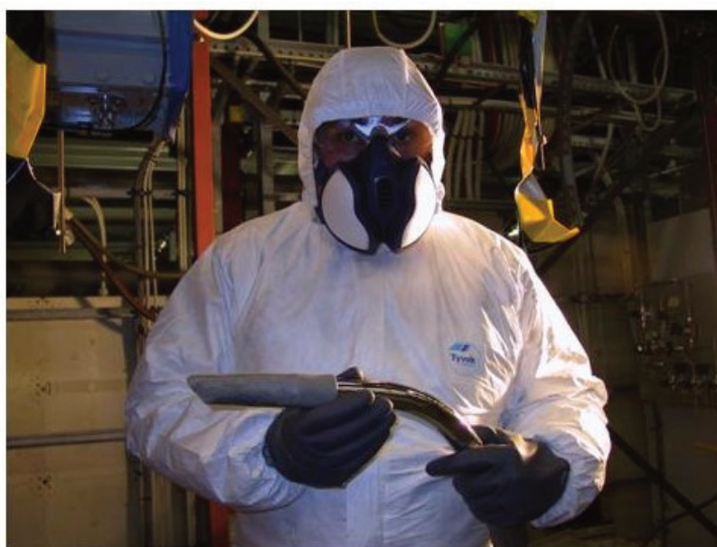
Fig. 9: Staff wearing protective clothing during work at SF_6 waveguides
