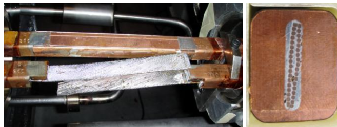
Fig. 1. (a) Main busbar interconnection splices in the LHC tunnel. The splice in the background is finished and in the foreground the two Rutherford type cables extending from the opposing busbar stabilizers are prepared for interconnection. (b) Cross section through a LHC dipole busbar. The Nb-Ti/Cu cable is electrically connected with the Cu stabilizer through the Sn96Ag4 solder alloy.
