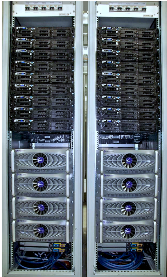
Figure 10. Storage manager nodes connected through Fibre Channel switches (QLogic SanBox 5600) to the NexSan SA-TABeasts (RAID-6 disk arrays).
