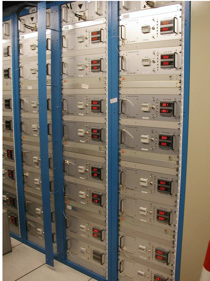
Figure 43. Photograph showing racks in USA15 housing the 280 V power supplies.
