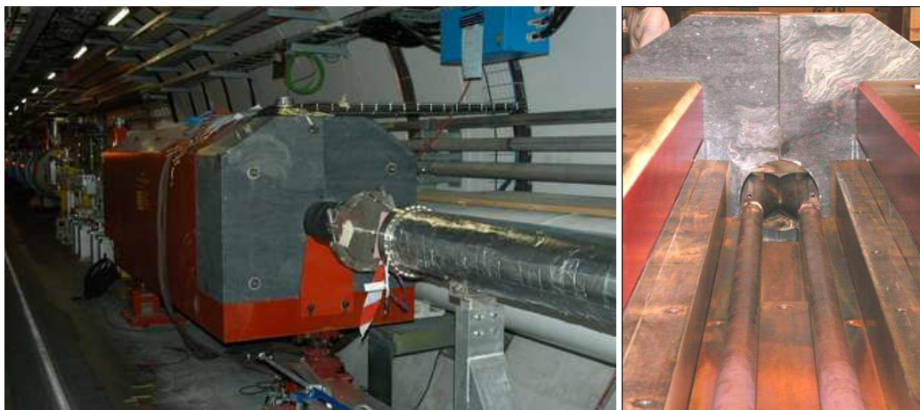
Figure 1.3: Photo of the TAN absorber located 140 m from the IP. Left: TAN fully assembled in the LHC tunnel seen from the IP side. Right: TAN during assembly at CERN seen from the top facing the IP. The 96 mm gap between the two beam pipes allows space for installation of detectors.
